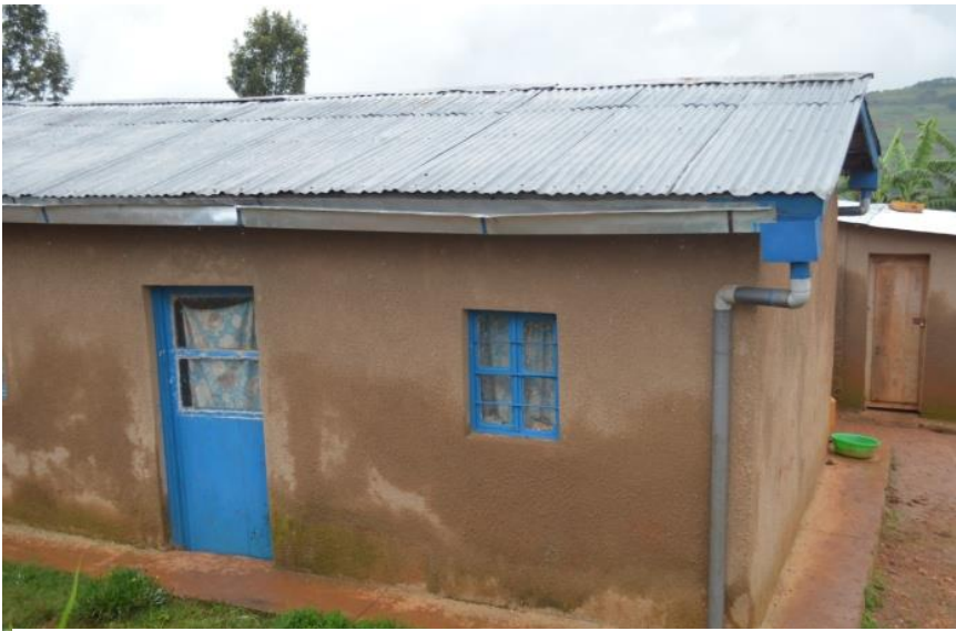
FIGURE 3-2 ROOFTOP RAINWATER HARVESTING
